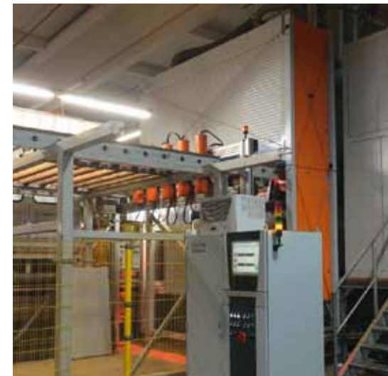
Installation in a production line
